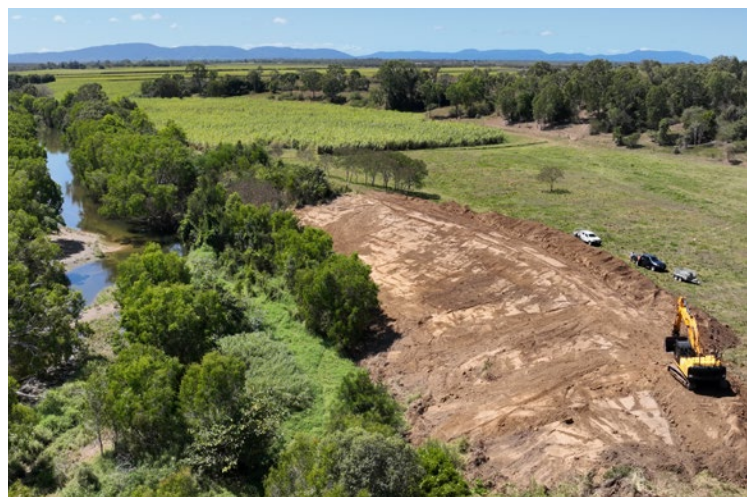
Figure 2 - Glassons site bank batter during works, installing physical structures that slow/direct water flow and catch sediment
