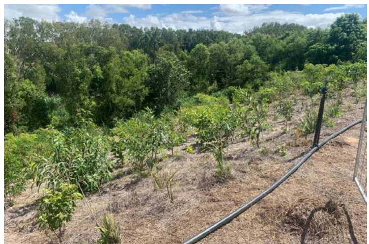
Figure 3 - Glassons site completed works following instillation of structures and planting of vegetation to further stabilise the streambank.
