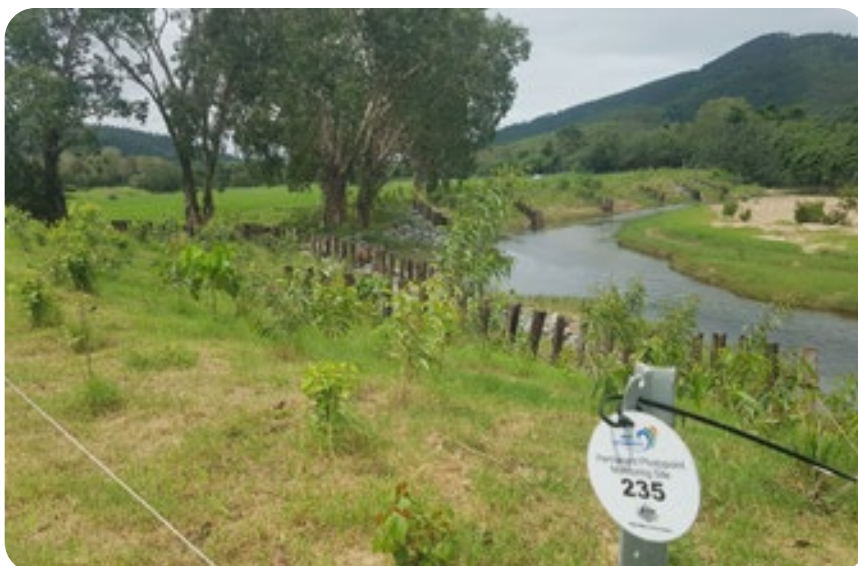
Figure 25: Before/After photo of works using permanent photo points to monitor the progress of streambank revegetation program. This site illustrates a great example of growth and uniformity of vegetation to develop bank stability.
