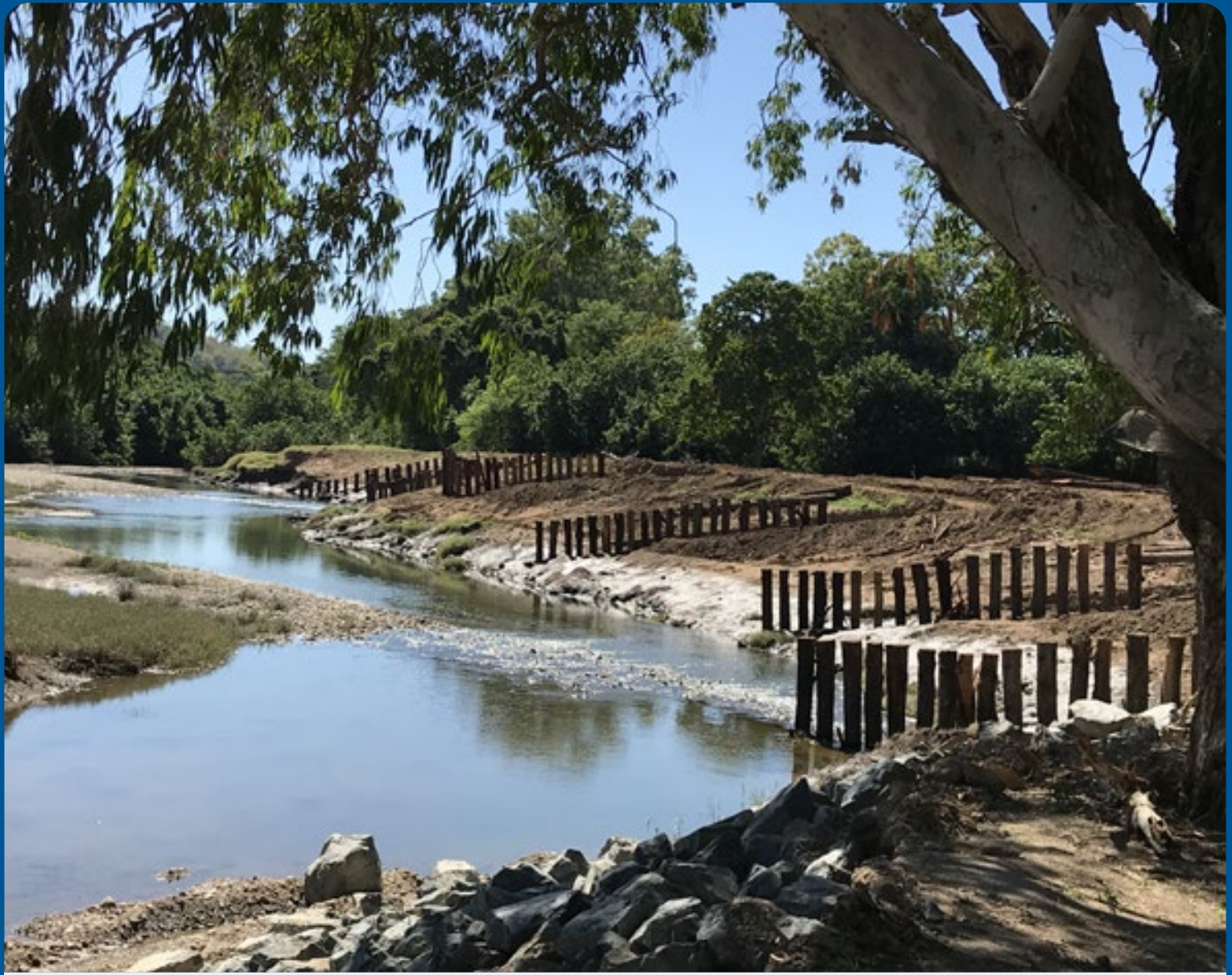
Figure 32: Photo of installation of timber pile fields on a property located in Mackay. Photo credit: Reef Catchments
