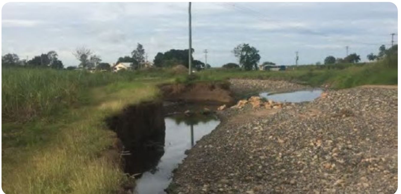
Figure 2: Photograph of damage on Oakey Creek from Severe Tropical Cyclone Debbie, causing threat to power infrastructure. The creek had little riparian vegetation along the banks. Photo credit: Alluvium Consulting
