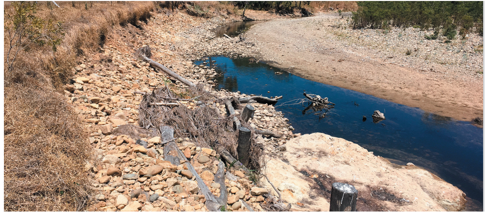
Figure 6 - Streambank erosion (Reef Catchments, 2021)
