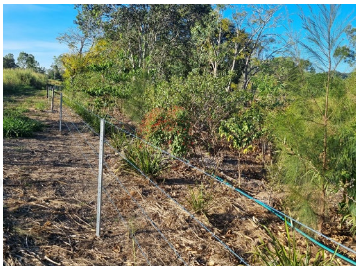
Figure 1 - An example of grazing fencing with a plain top wire installed in the Mackay Whitsunday Isaac Region
