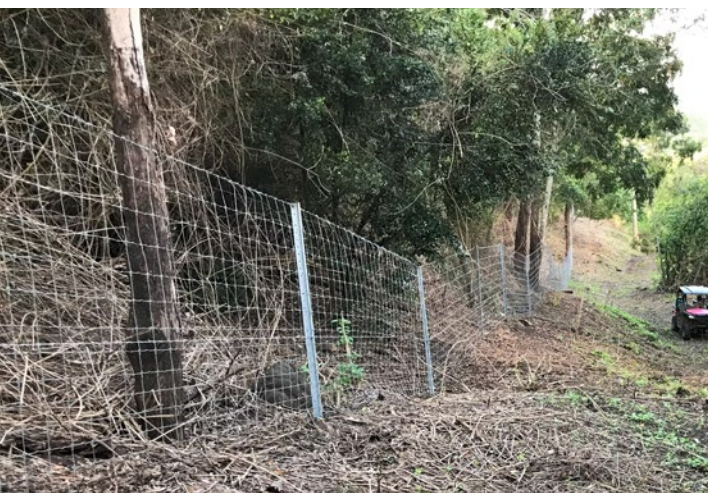
Figure 2 - An example of goat fencing installed in the Mackay Whitsunday Isaac Region
