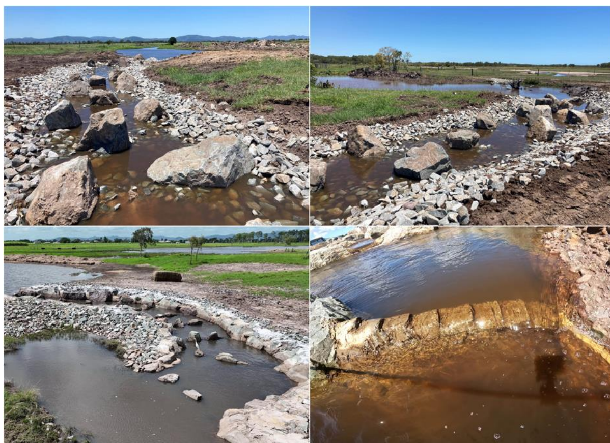
Figure 2. Top - Looking upstream (left) & downstream (right) at Alligator Creek wetland fish passage works; Bottom - Showing Macs wetland rock ramp fishway (left) & the nursery slot (right) incorporated into the design.
