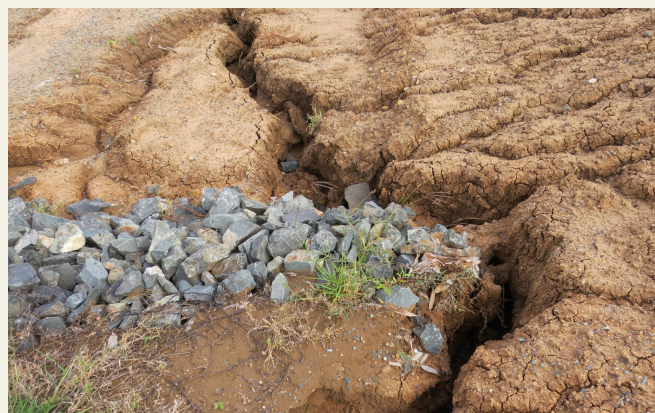
Image 1: Failure of a rock check dam in a sodic clay soil.
