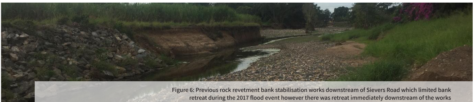
Figure 5: Near vertical bank between 2–3m in height which is actively eroding as part of a meander migration process and threatening an electricity pole adjacent to Oakenden School. Remnants of rock bank protection works which were outflanked during the 2017 event remain in the channel
