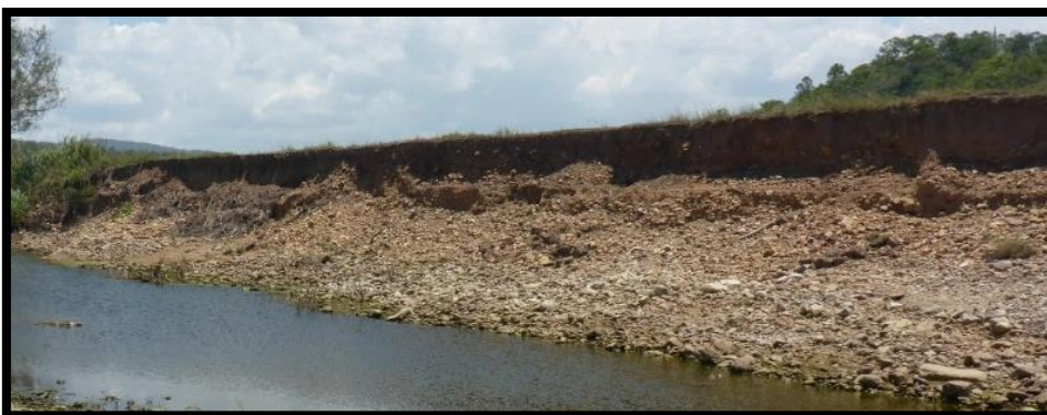
Figure 2: Erosion at WH3, Nov 17
