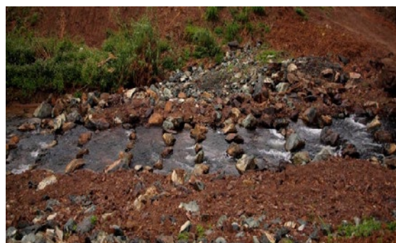
Rock-ramp fishway constructed at the Biggs Road culvert - restoring passage and flow for fish migration through the Proserpine River Main Channel
