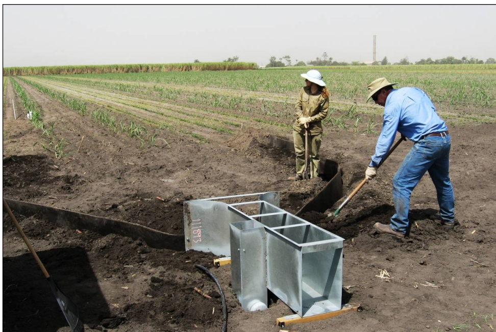
Figure 6. Installation of Marian Soil strip scale water quality monitoring equipment.
