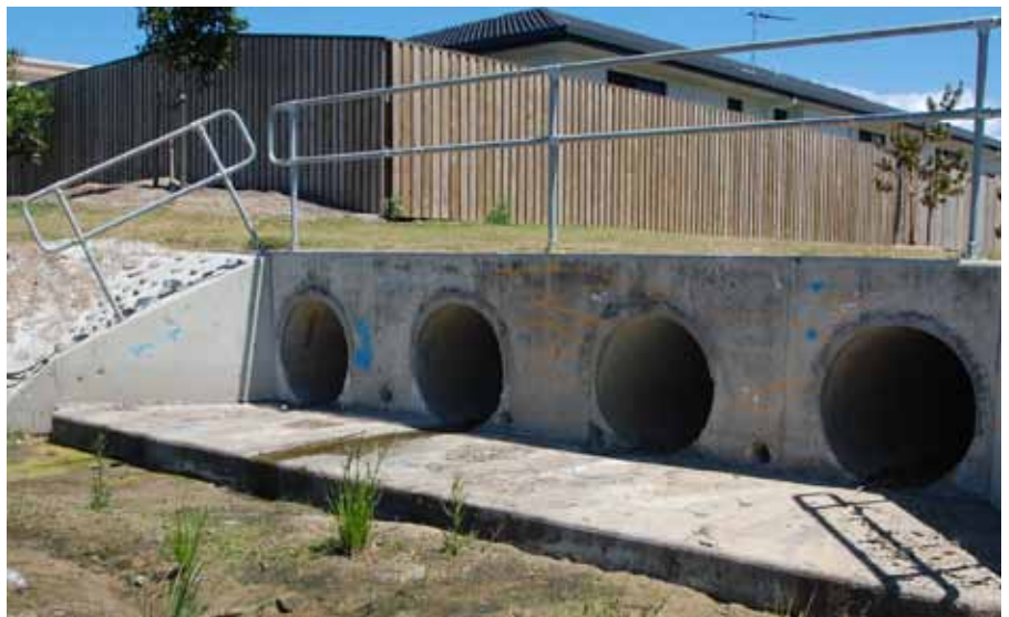
Storm water outlet at Cuttersfield Estate, Ooralea.
